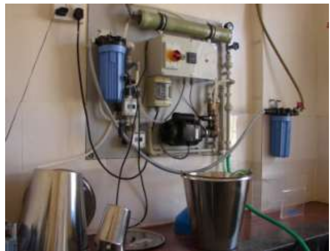
De-ionising equipment in the infusion room
