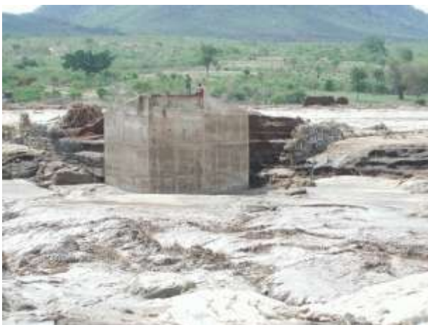
The bridge washed away by flooding
