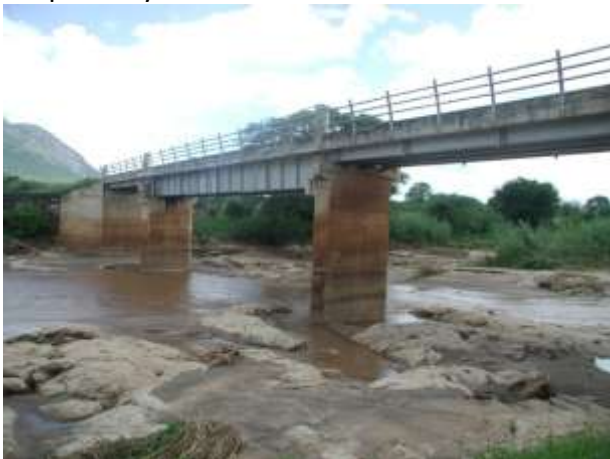
The bridge before the flood
